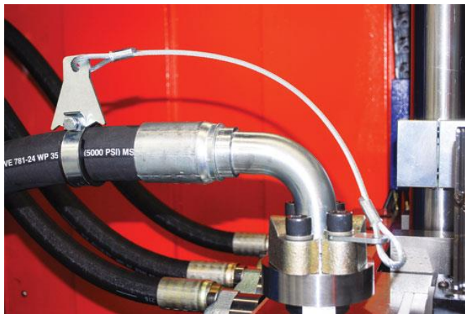
Figure 10: Example of hose whip cables and securing method
