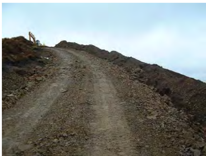
Figure 21 Example of an insufficient site road, due to:
