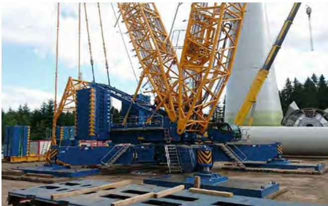
Figure 2: 650 ton Pedestal Crane
