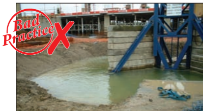
EXAMPLE OF A FLOODED TOWER FOUNDATION
