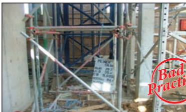
POOR ACCESS TO THE CRANE MAST
