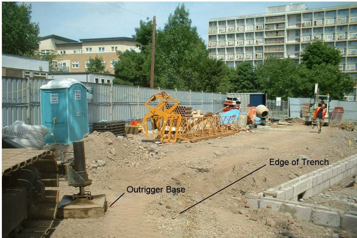
Excavation too Close to Outrigger and Track (See 5.3)
