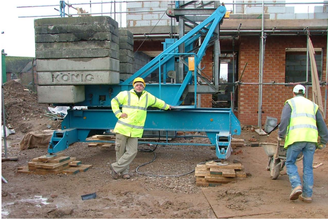
Lack of Base Fencing (See 5.2)
