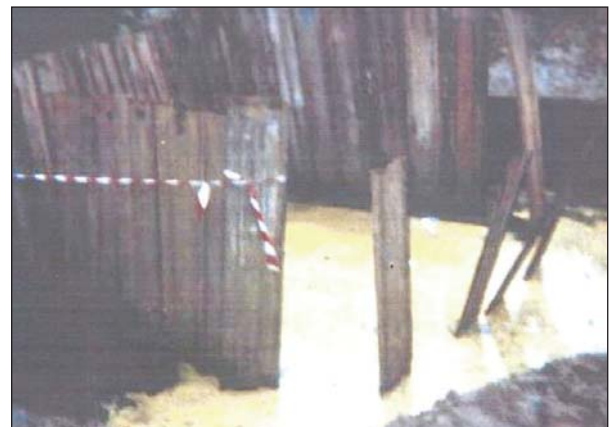
Figure 1.5 A flooded excavation
