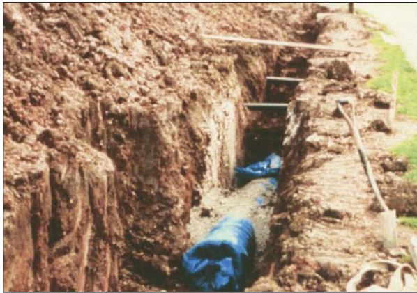
Figure 1.6 Examples of excavation surcharges and lack of support
