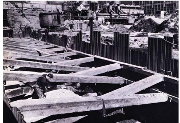
Figure 2.02 Fabricated trench shoring- wooden struts and walers in combination with trench sheeting
