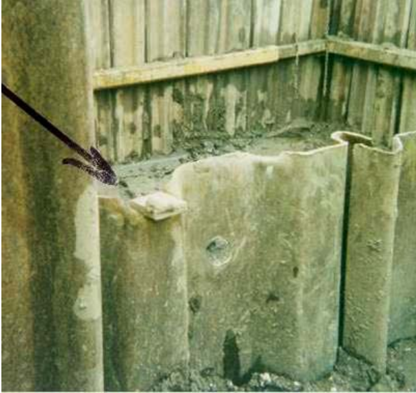
Sheet Damage by Chain Hook
