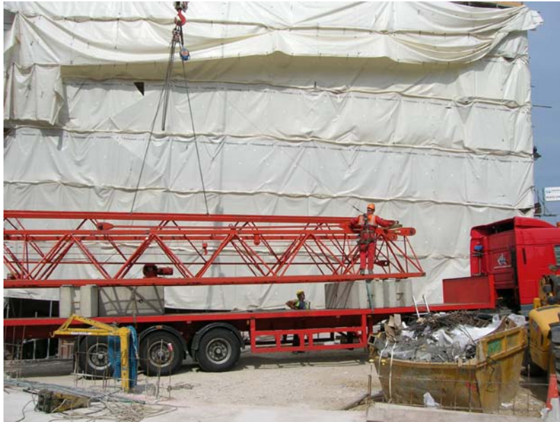
Example of Poor Practice
