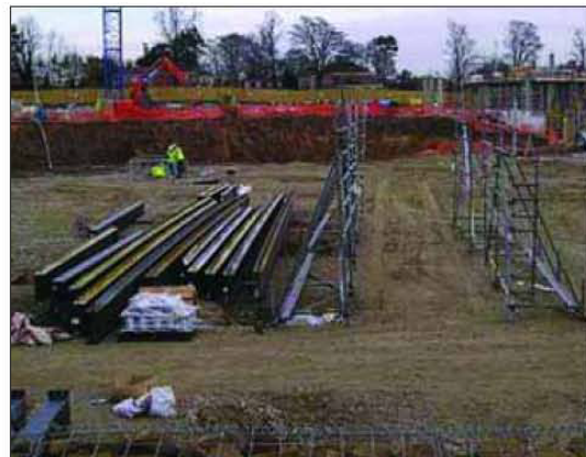
Figure 1 Drive through unloading gantry
